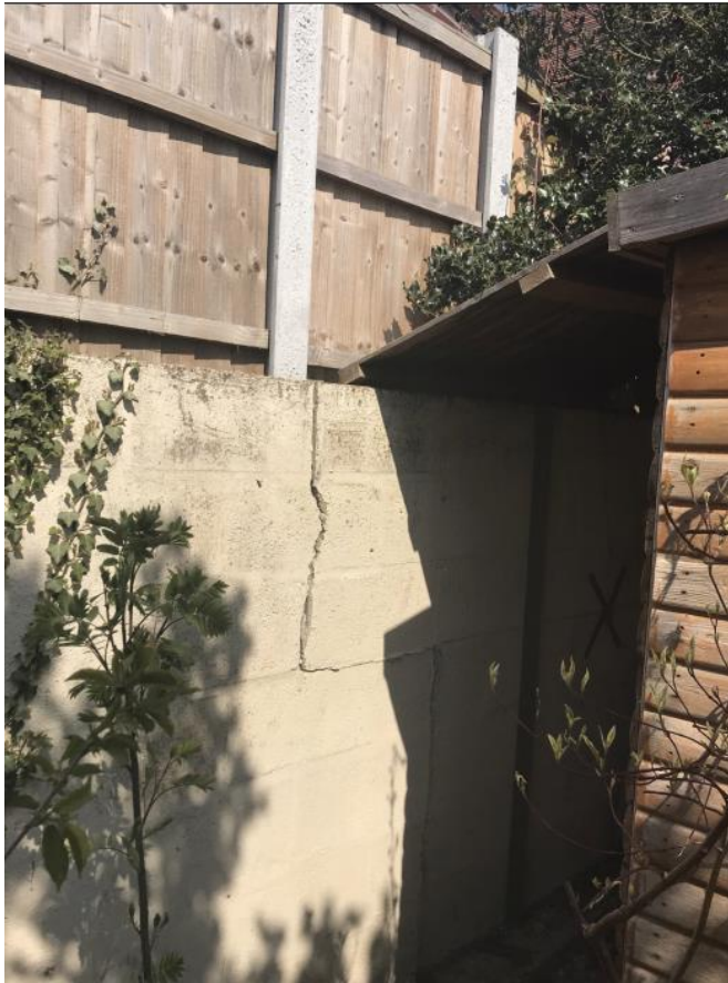
figure 27: The cracked boundary wall plot 6 / White Horse House
